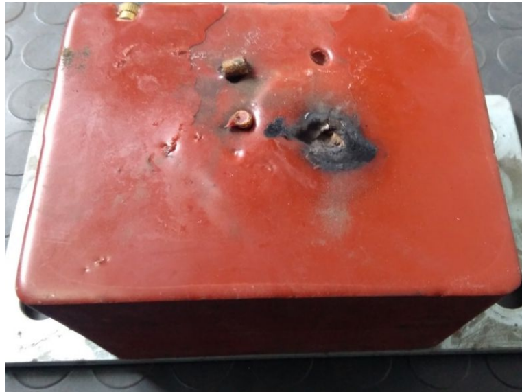
Damaged CT Found in Panel
