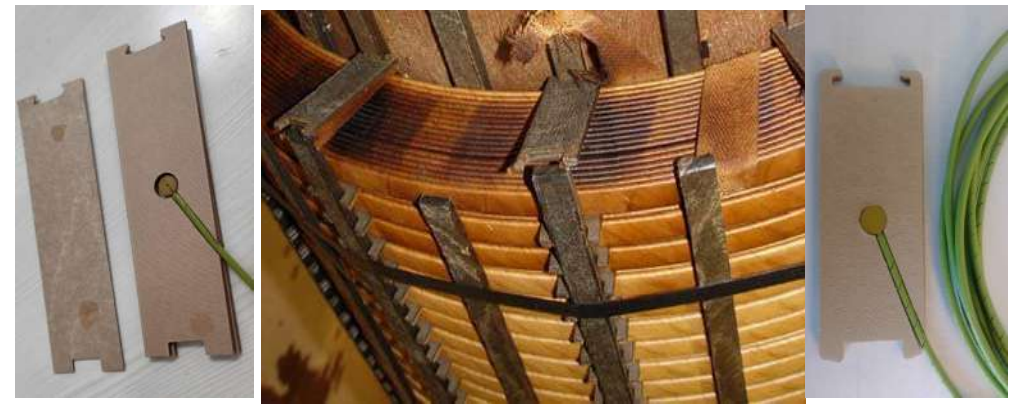
Fiber Optic Temperature Sensors installed on the Spacer
